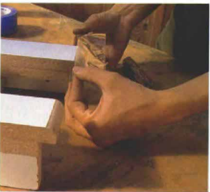
Sealing edges and joints. Sealing the edges creates a smoother concrete finish. After the exposed edges of the sink knockout are coated with spray adhesive (top photo), the porous substrate is sealed with packing tape (bottom photo).
